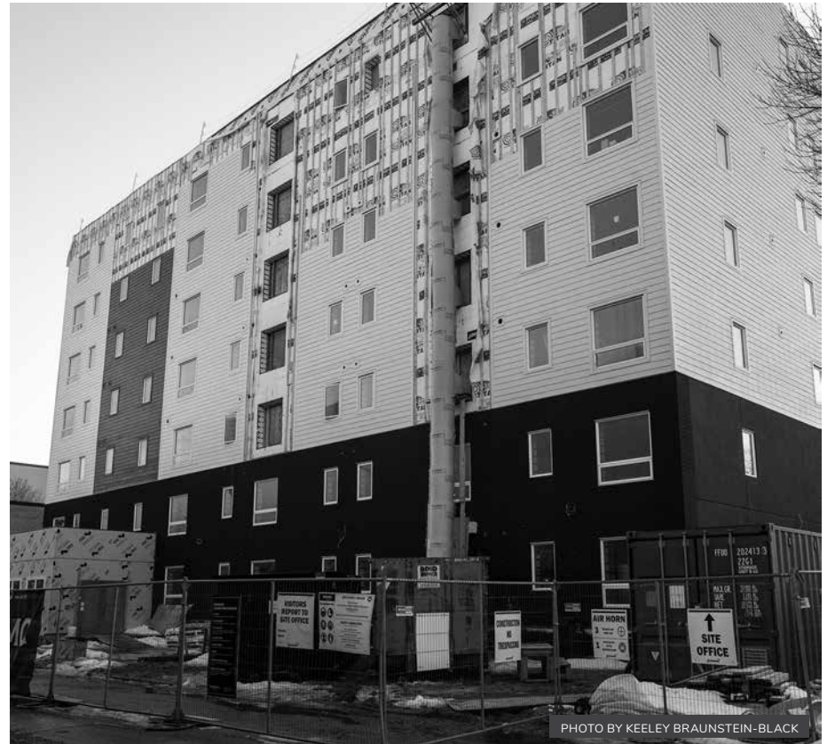
This building under construction at 380 Young St. is owned by the Opaskwayak Cree Nation.
