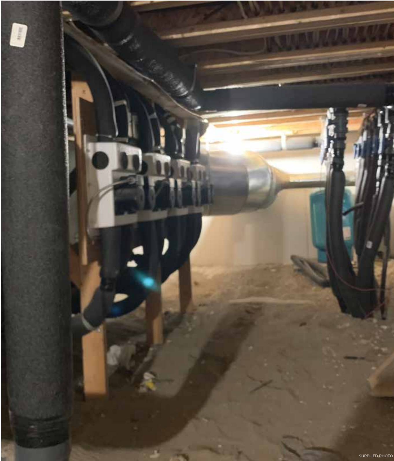
Geothermal piping in a residential home. Manitoba climate advocates say that replacing natural-gas heating with geothermal heating is essential to lowering the province's emissions.
